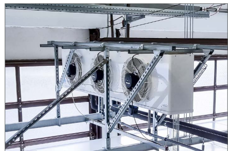
Machine room conditioning
