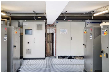
Switch cabinet with S7 controller
